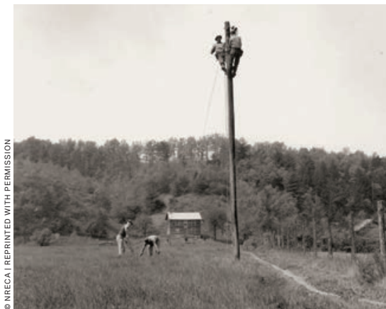
Powering the Frontier: Linemen install an electric pole in Texas in the olden days.
